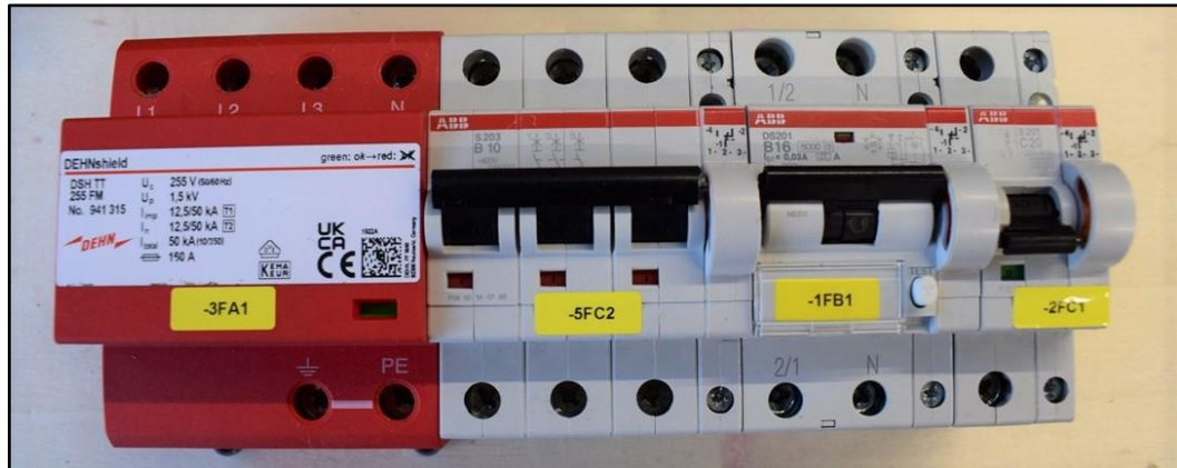
Fig. 14 Lightning protection and circuit breakers in ControlShield central rear
