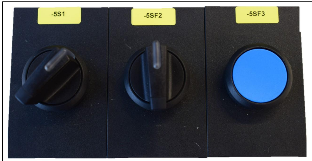
Fig. 12 Controls 5S1, 5SF2, 5SF3 in ControlShield right centre
